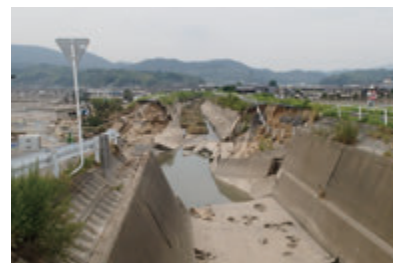
高馬川の堤防決壊箇所(2018 年倉敷市真備町) Dyke breaching of Takama River (Mabi-cho Kurashiki, 2018)
